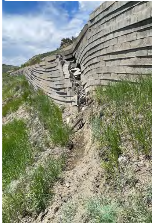
US 50 Cerro Summit Landslide/Wall
